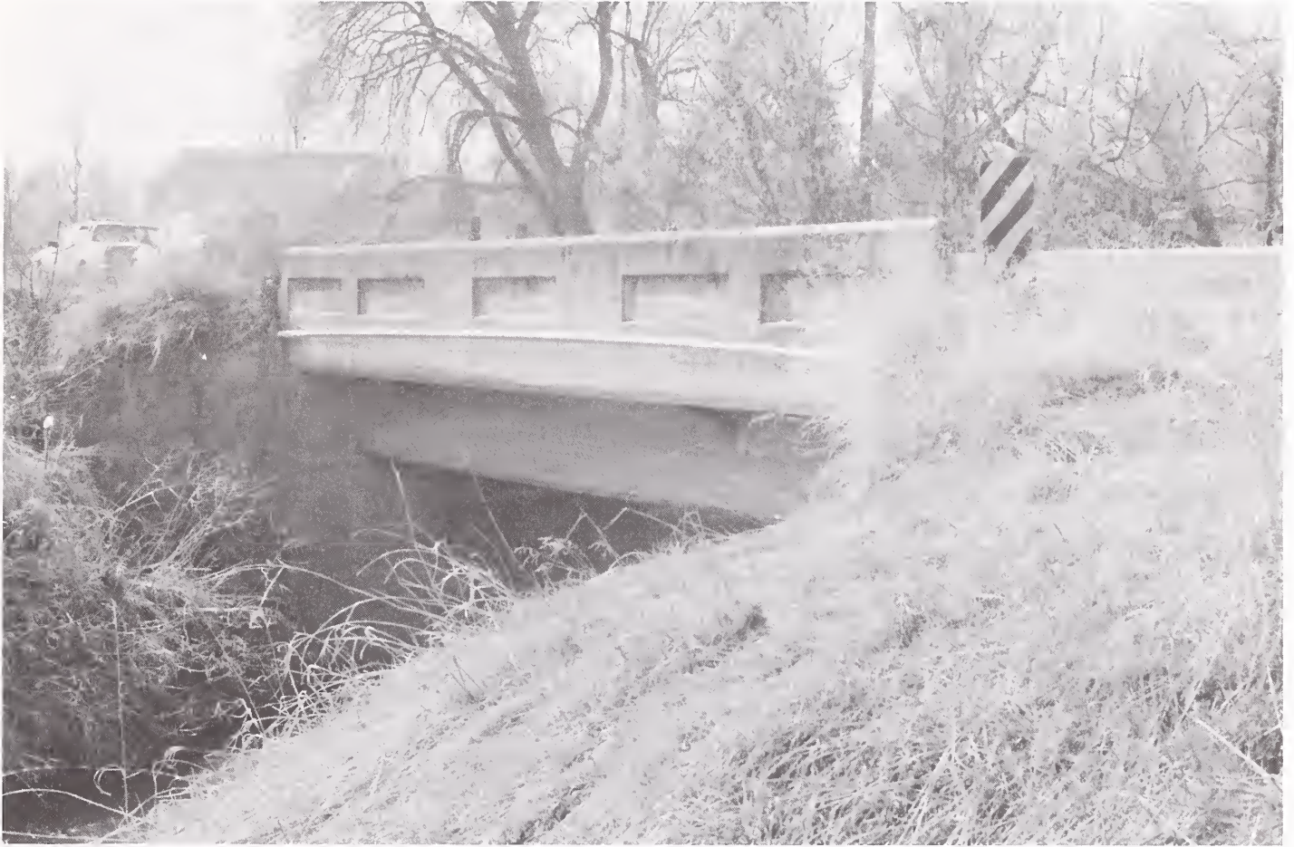
The Bluewater Creek Bridge in Carbon County. Constructed in 1913, the structure was the first reinforced concrete T-beam bridge built in Montana.
